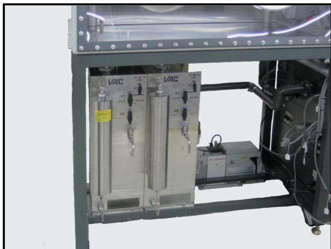
Under Glovebox Installation
